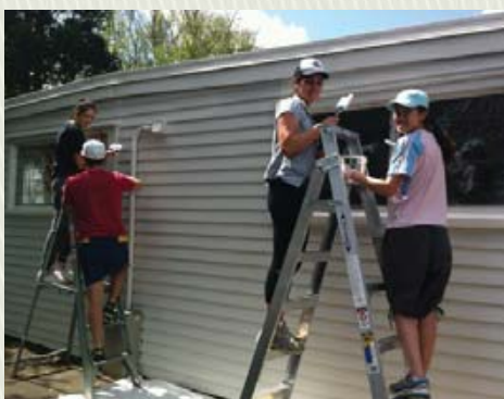
KPMG staff personally adding in their support by helping to paint the exterior of Edmund Hillary School.
